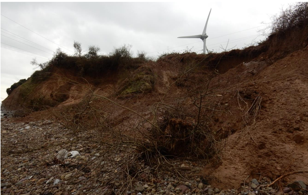
Figure 15 Area of collapse showing flatter slope
